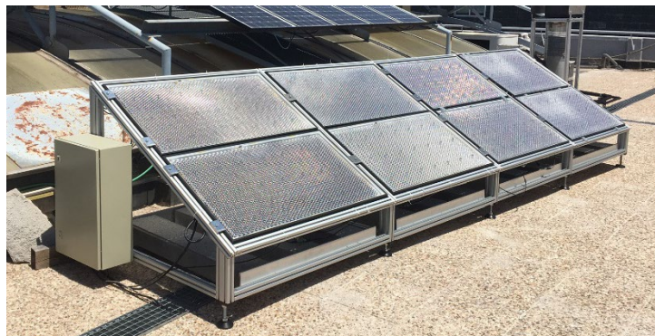
Figure 3: 8 module pilot installed at the IES in March 2021. The four outer panels are Gen2 translucent panels. The four inner panels are Gen1 hybrid panels.
